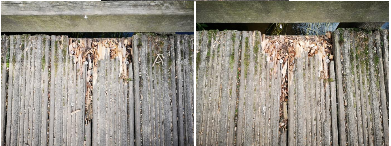
MID-POINT FACING UPSTREAM - WET ROT TO TIMBER DECKING. (SEE DIAGRAM POINT 3).
