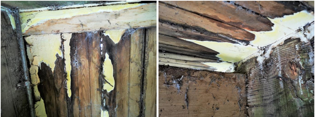
MID-SECTION - EXAMPLE OF YELLOW MOULD TO DAMP AREAS.
